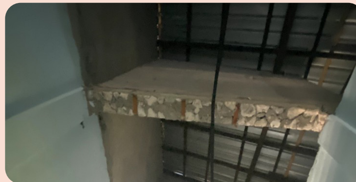
A dangerously unsafe reinforced concrete beam that was made with coral aggregate.
