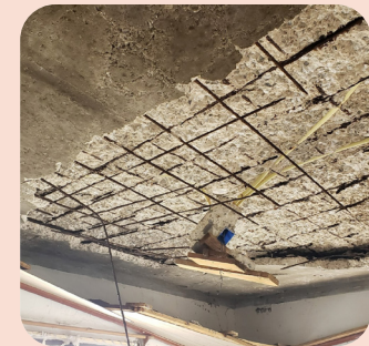
A dangerously unsafe concrete slab made using beach sand
