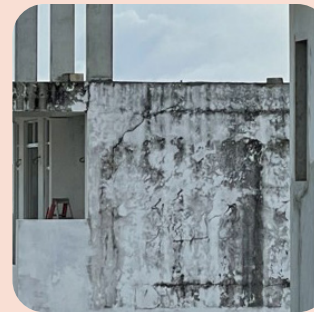
A wall plastered with plaster made from beach sand that has badly deteriorated.
